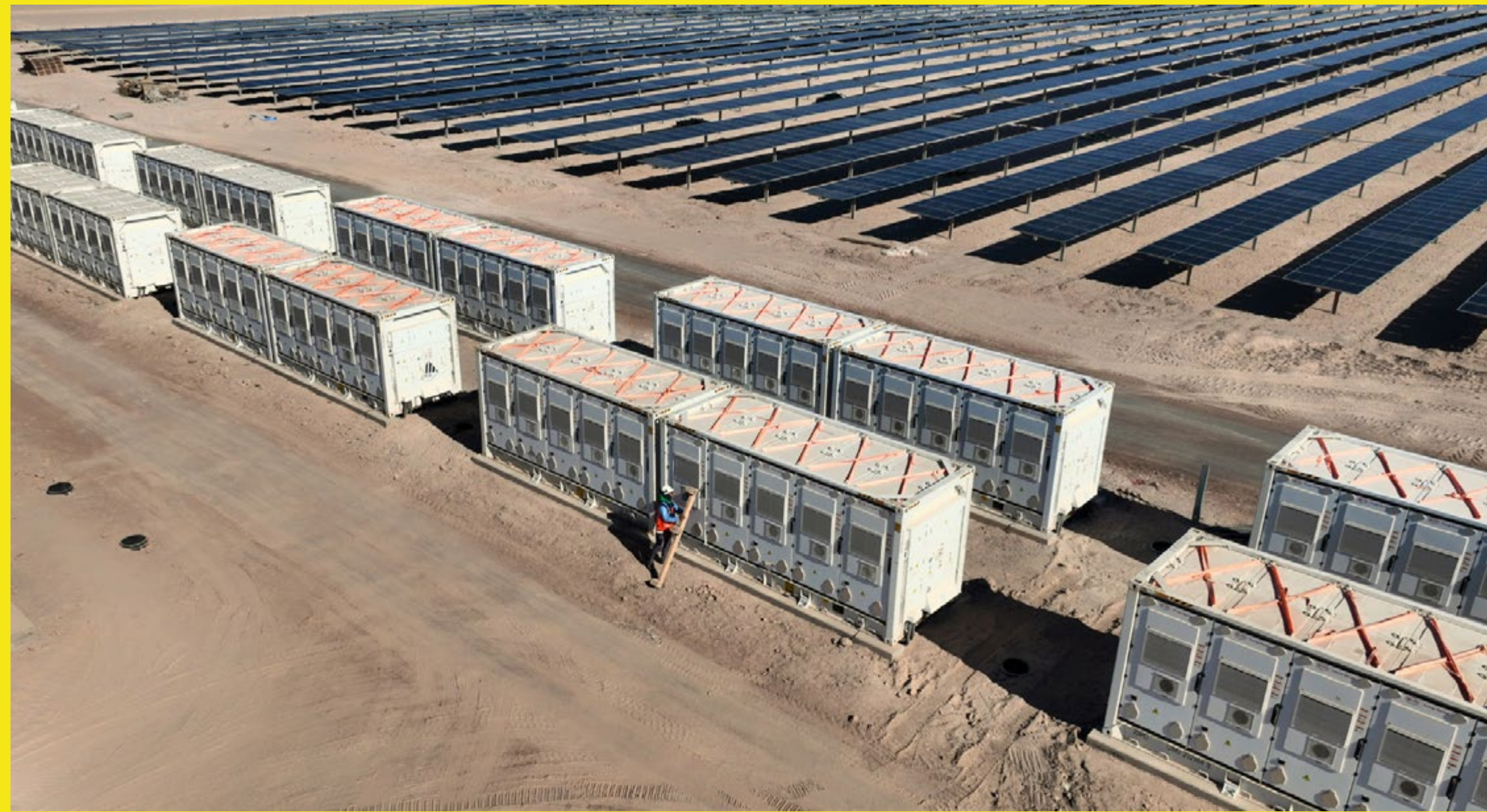
Elena 446 MW + 3.5 GWh hybrid plant, Chile
