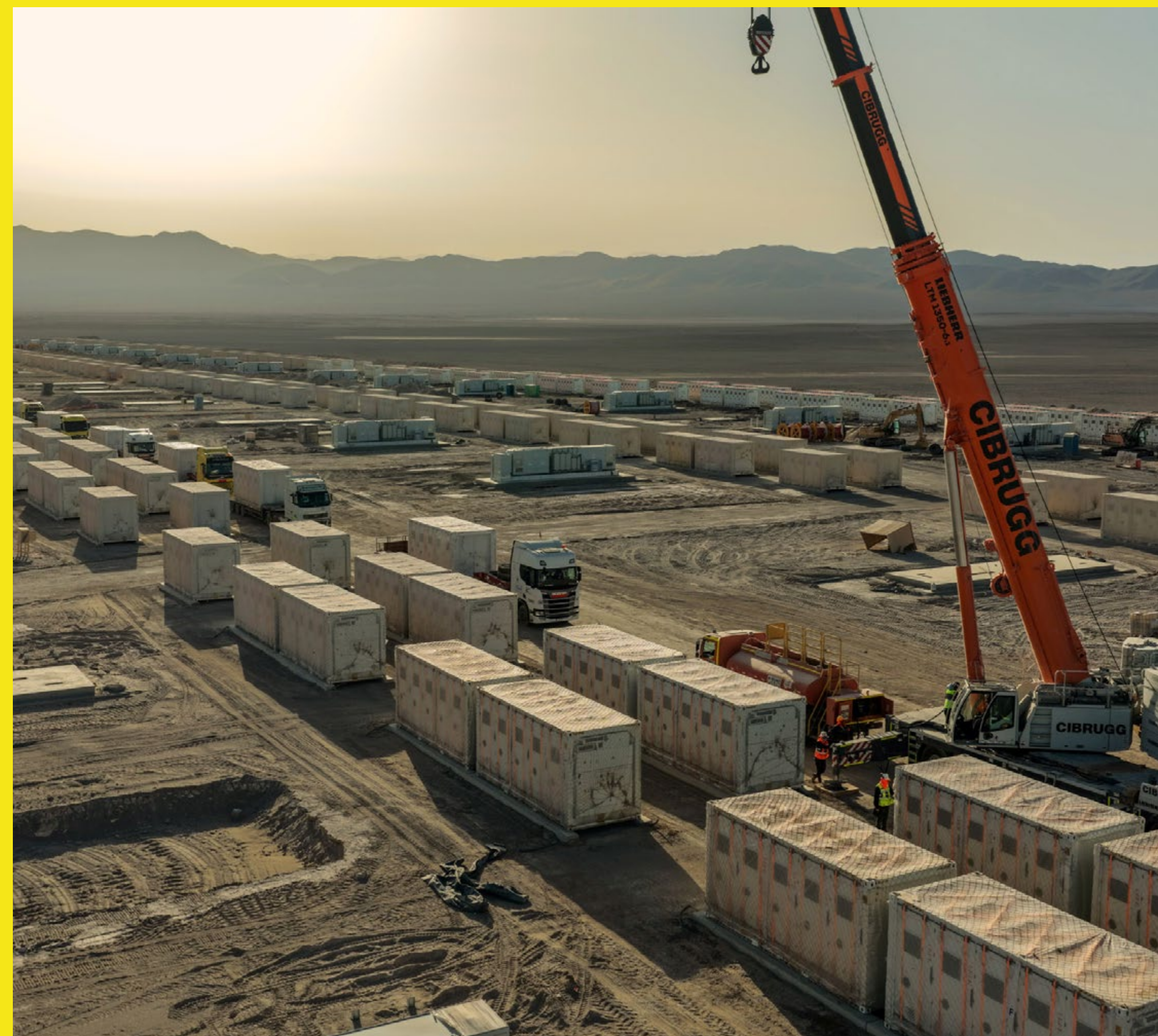
Elena 446 MW + 3.5 GWh hybrid plant, Chile
