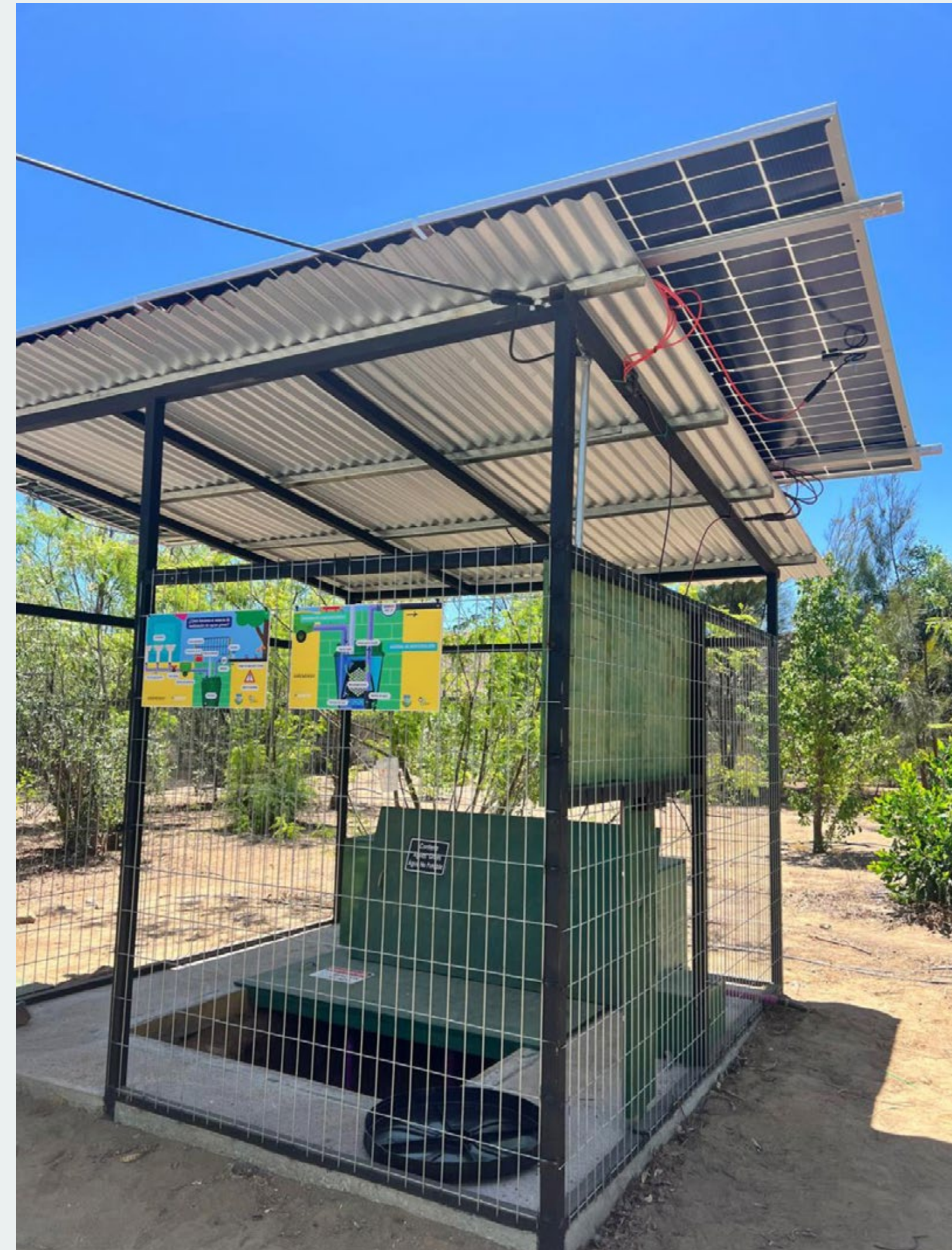
Solar panel-powered pump
